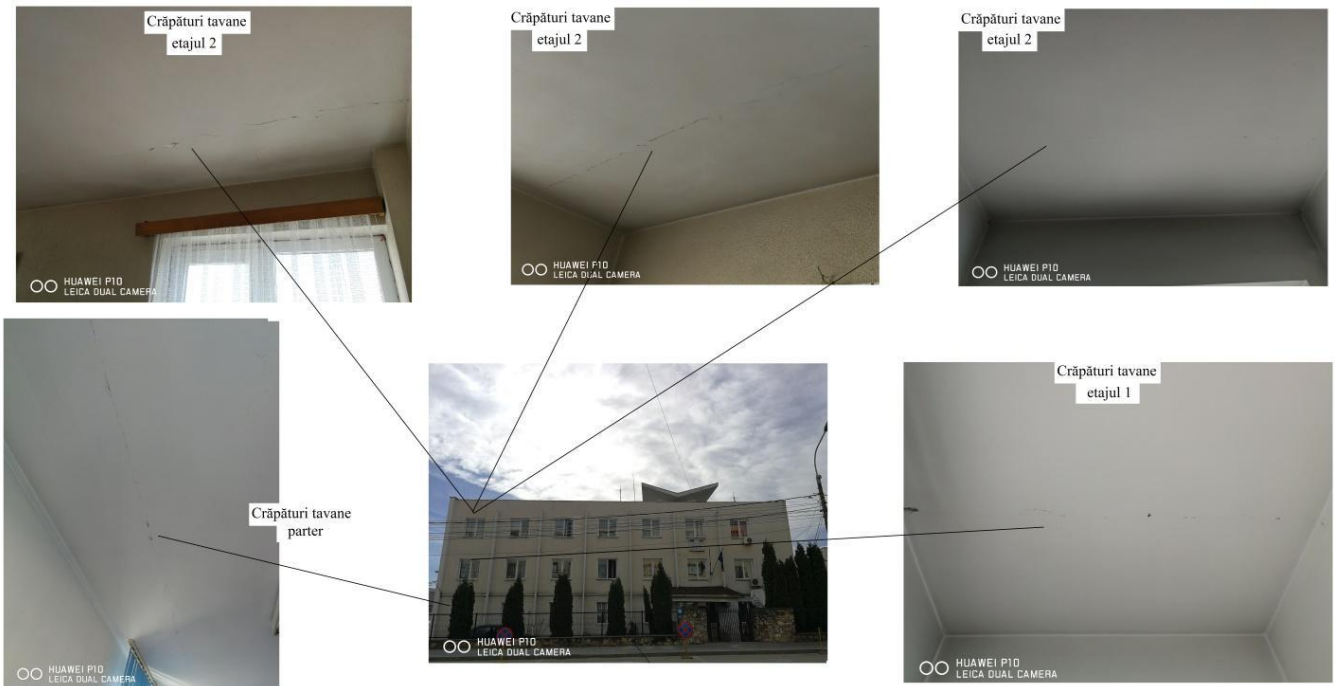
Fig. 4 - The floor is cracked in several areas of the building and there is a risk of collapsing
