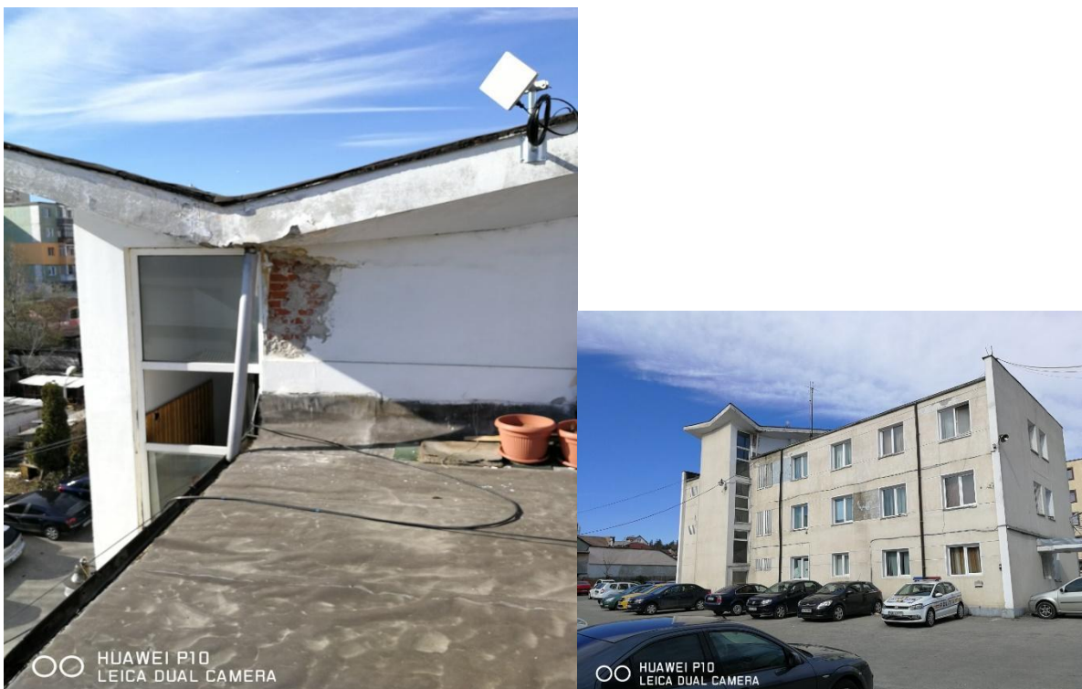
Fig. 5 - The façade is damaged and has never been repaired
