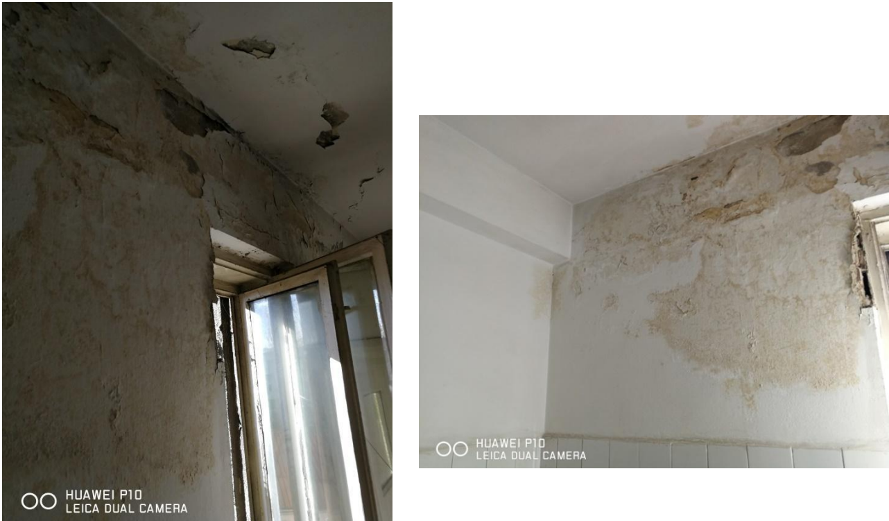
Fig. 6 - There is extended damage on the interior due to water infiltration
